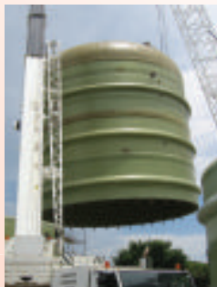
CORROSION-RESISTANT PIPE AND TANKS
